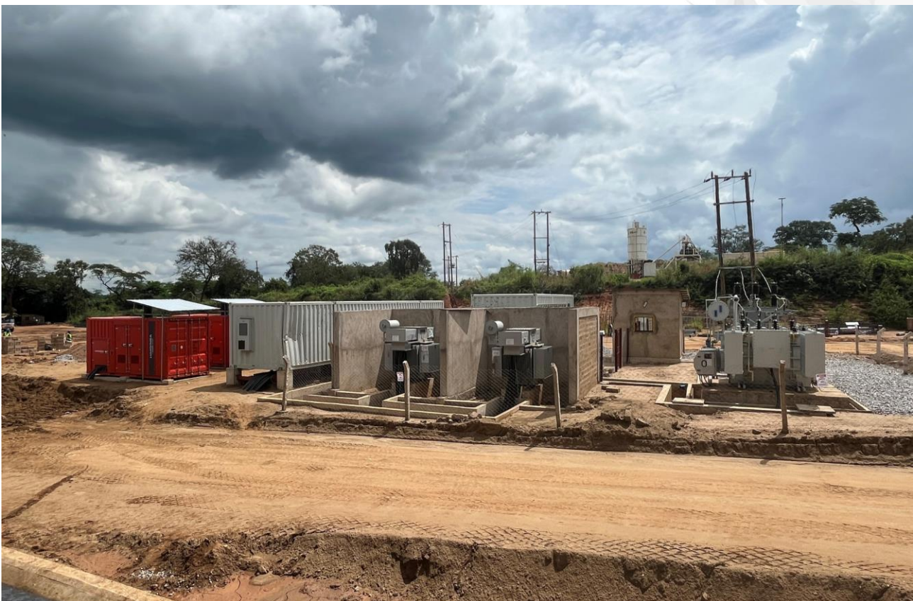
Figure 1: Transformer yard and backup generators at the Lindi Jumbo Graphite Mine.
