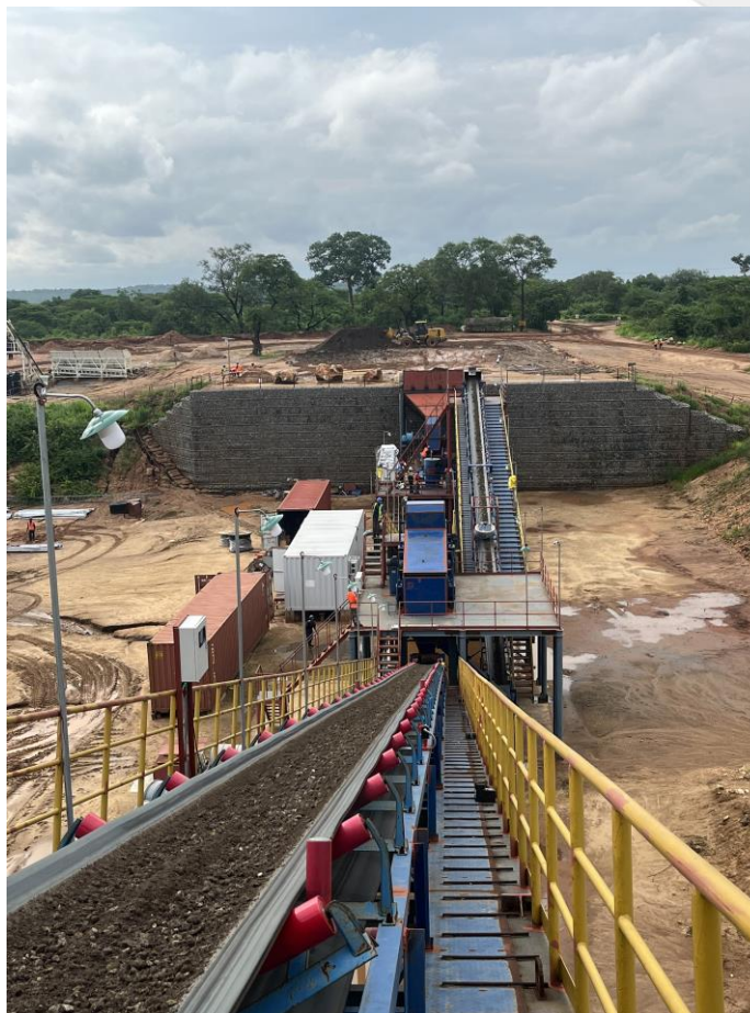
Figure 4: Crushed ore on Conveyor 003 on the way to the fine-ore bin during crushing operations in January.
