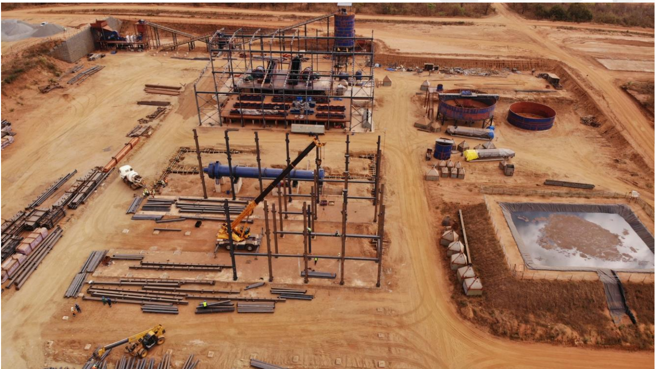
Figure 2: Steel frameworks of the Drying & Screening building (foreground) and Concentrator building (background) as at the end of September 2023.
