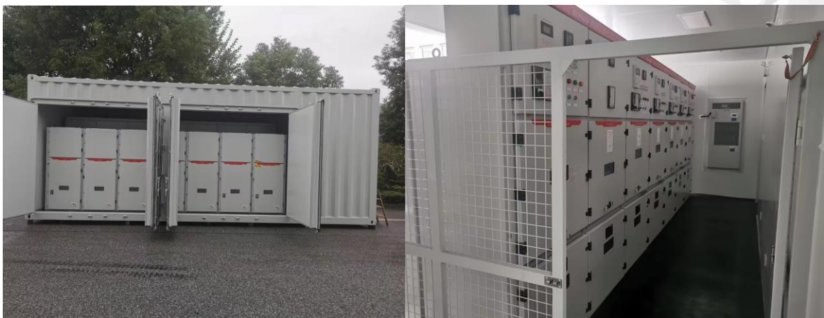
Figure 3: Containerised 11 KV Switchgear & 400V PCC Cubicles en-route to Tanzania.
