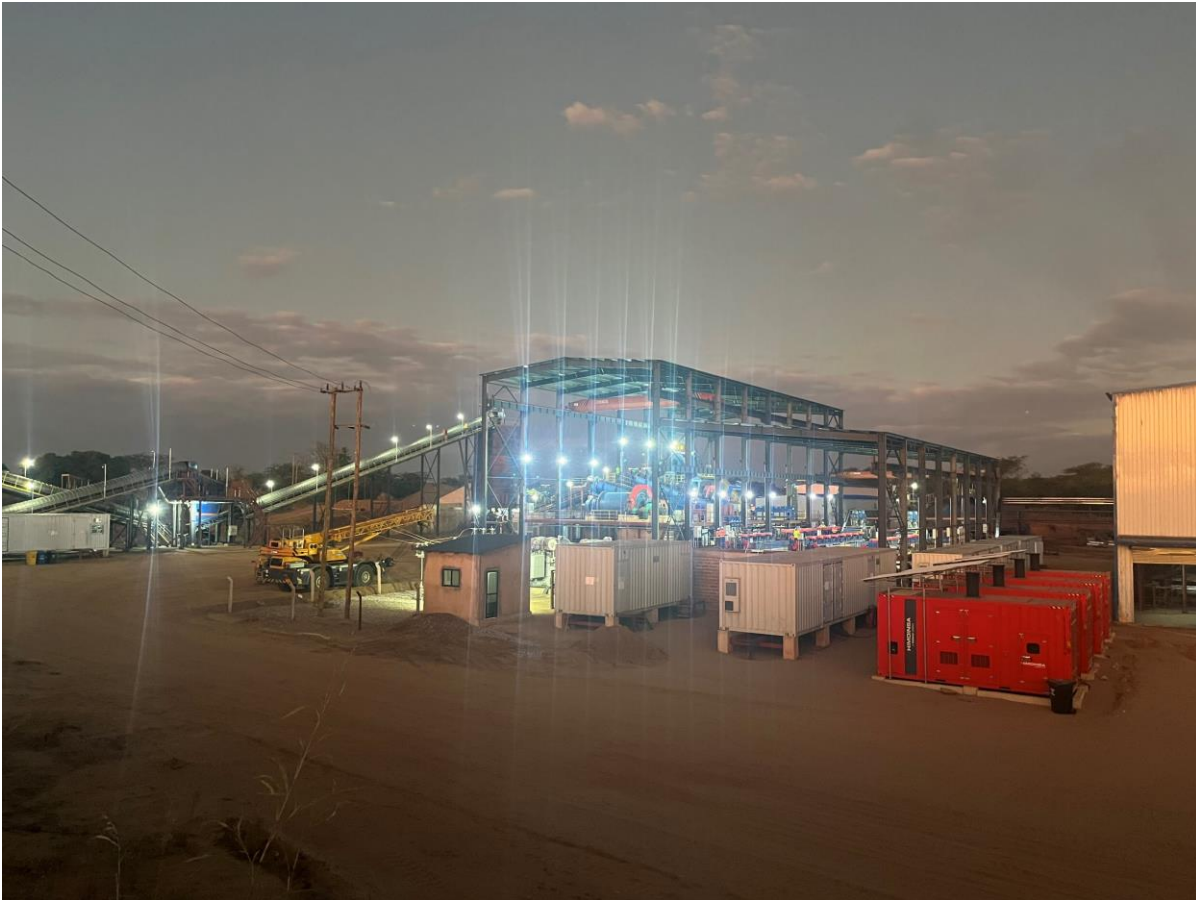
Figure 1: View of the concentrator section during nightshift.
