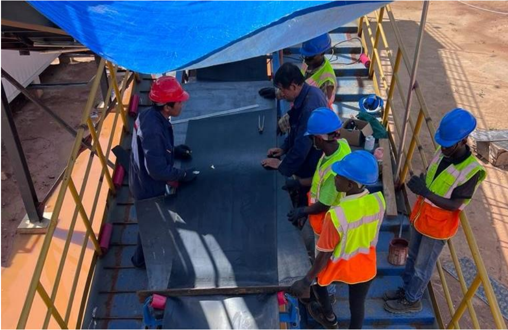
Figure 1: Recent Belt splicing activity at the Crushing Circuit, prefacing Imminent Dry Commissioning
