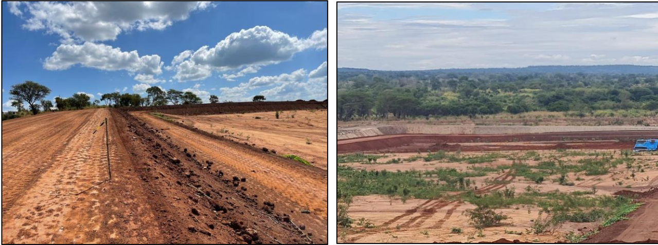
Figure 2: Completed clay-lined embankment walls (left) and in progress (right) of the pre-depositional area of the TSF in preparation of the installation of the HDPE liner.
